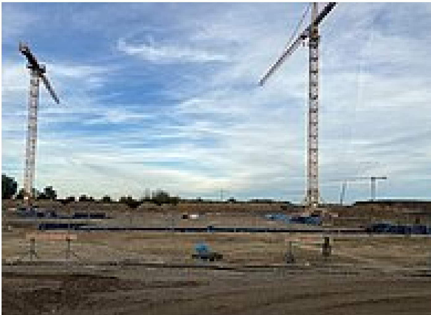
Large construction site: the construction ground of the sewage sludge utilisation plant in Berlin-Waßmannsdorf in October 2022
