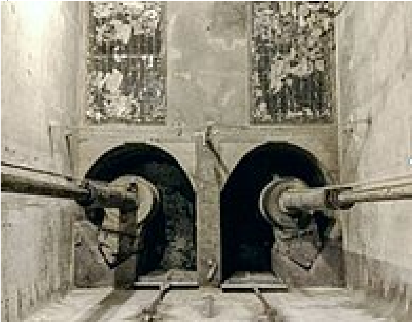
The previously installed shredder at the La Crosse wastewater treatment plant.
