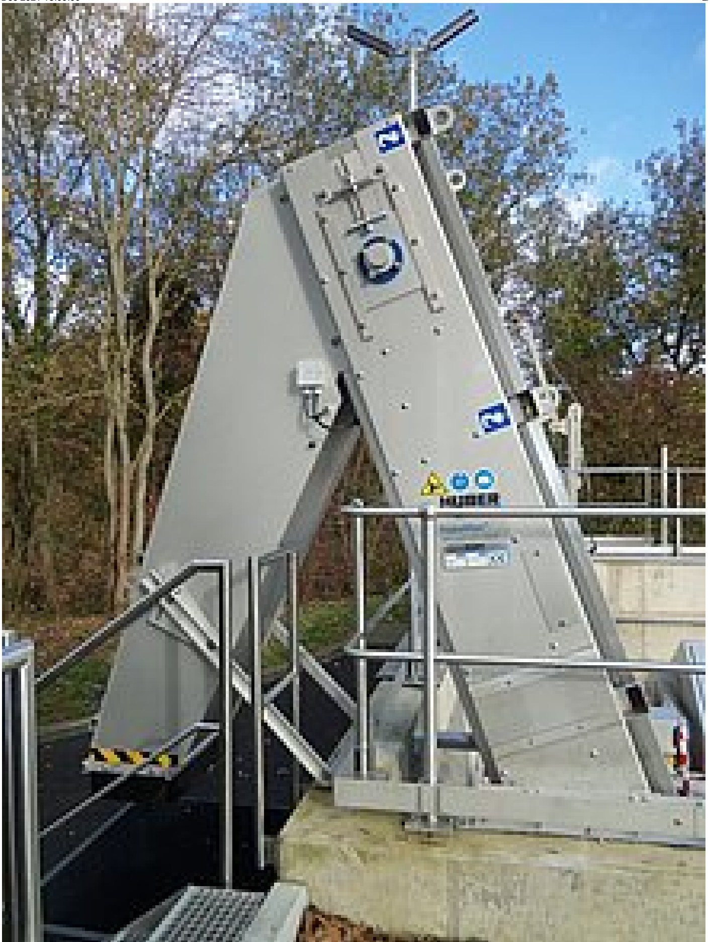
In-channel installation of a RakeMax®-J screen on STP Aachen-Horbach
