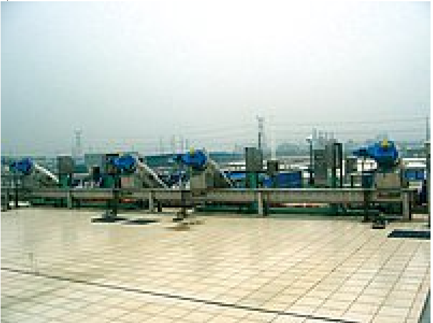
Four of the ROTAMAT® Fine Screens Ro 1 / 2200 installed on WWTP Zhuyua
