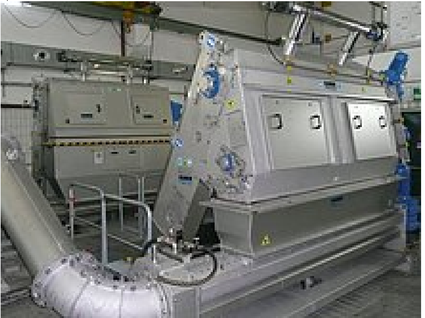
Back view of line 1
