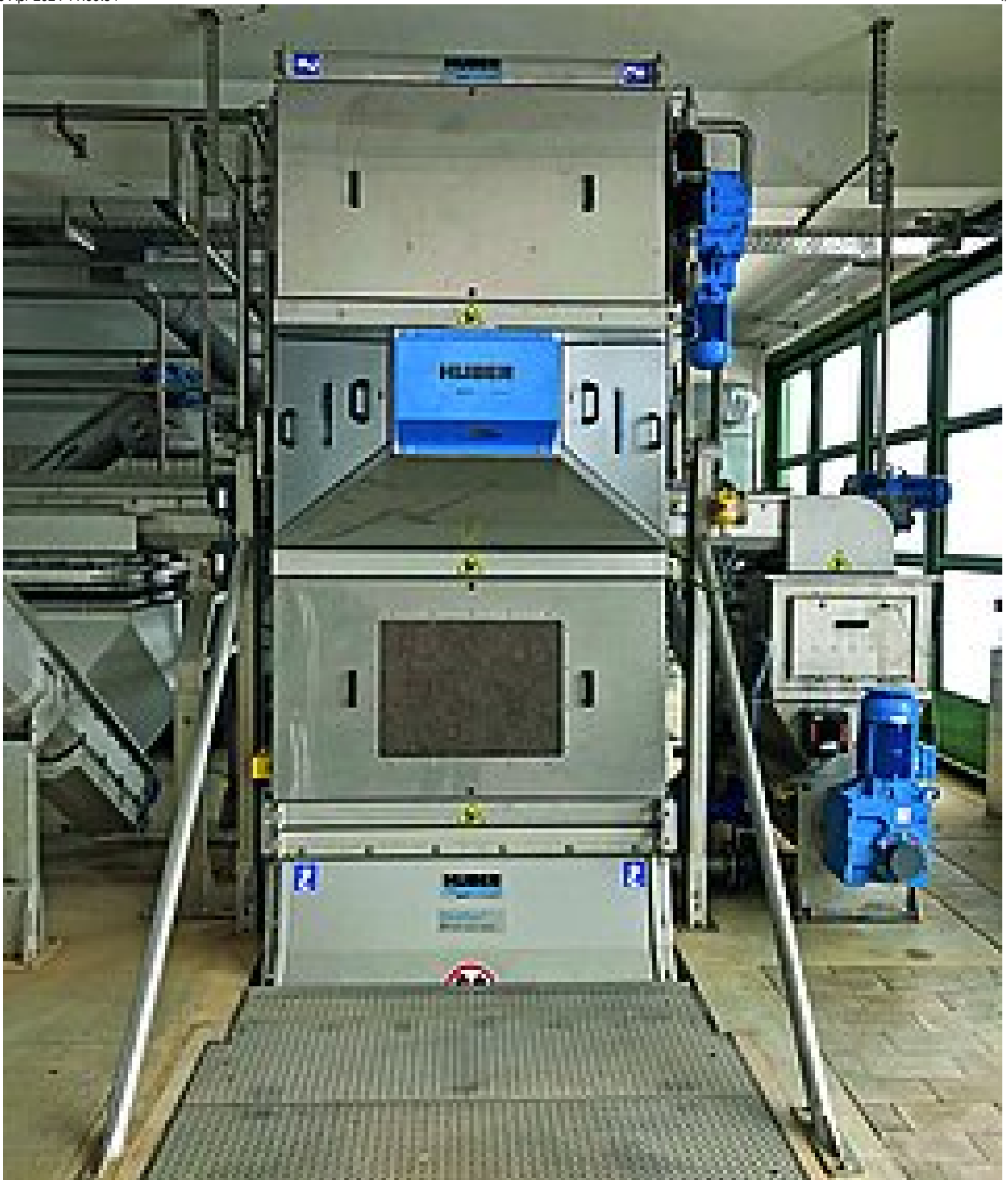
"Safety Vision" installation, running to the full satisfaction of the plant operators
