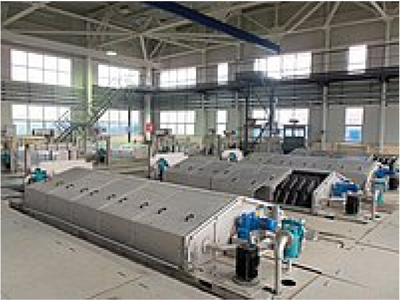
RoDisc® Rotary Mesh Screens at the plant
