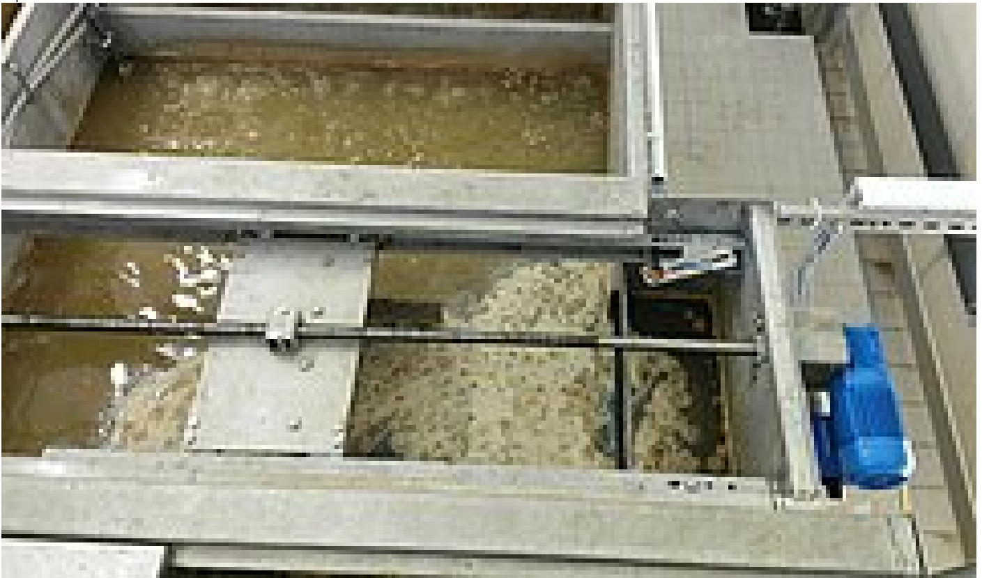
Fig. 2: New grease chamber with grease paddle in action
