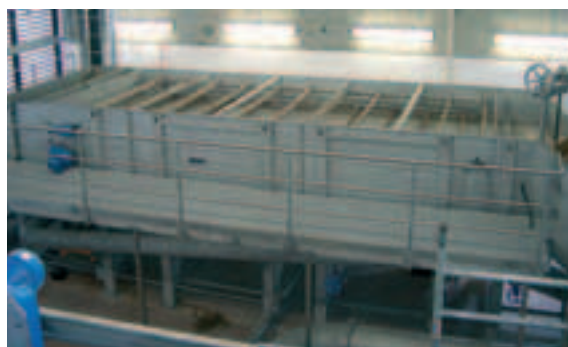
HUBER Dissolved Air Flotation Plant HDF without chemical treatment stage for up to 400 m 3 /h
