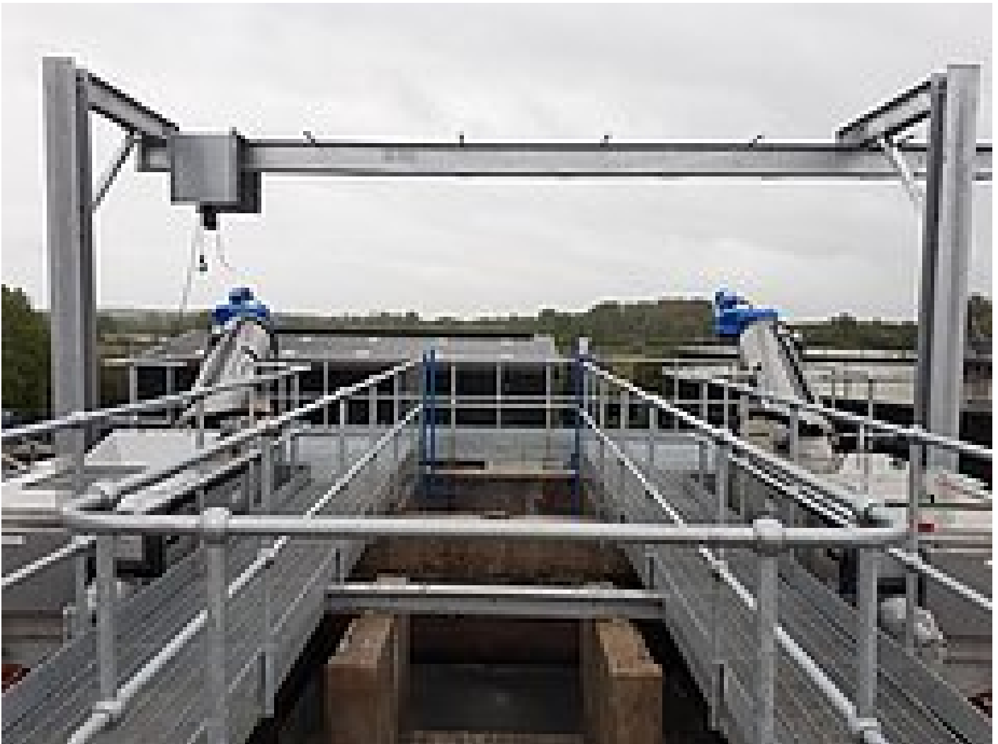
2x HUBER Sludge Acceptance Plant ROTAMAT@ Ro3/1200/355 units installed at Wanlip STW
