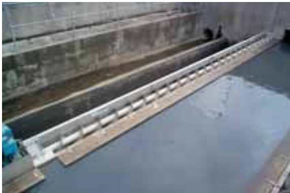
HUBER ROTAMAT® Screen RoK 1 installed in a storm-water discharge channel
