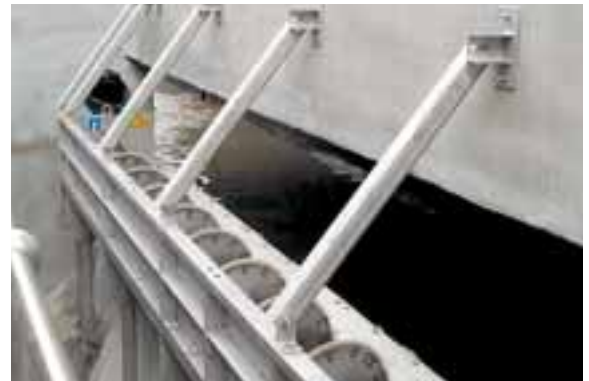
HUBER ROTAMAT® Screen RoK 1 installed at a overflow sill
